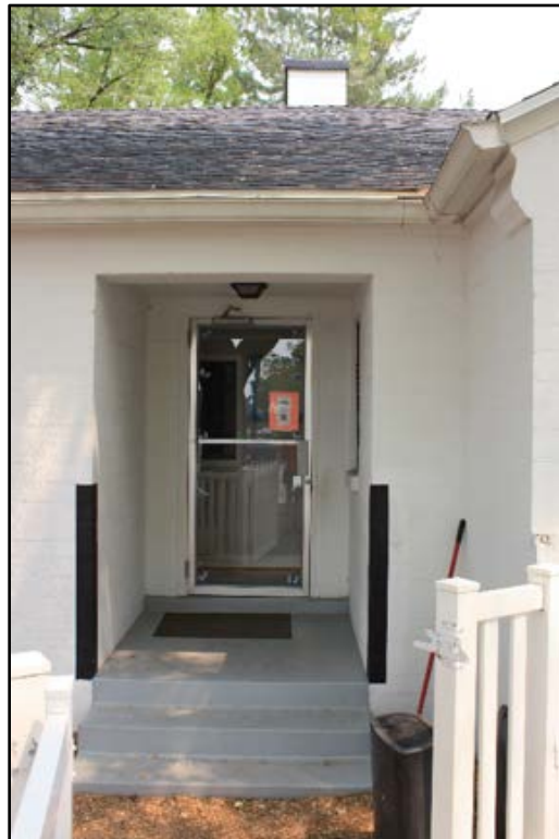
Photo 4 of 54. Entrance into the west addition with typical aluminum glazed door. Camera facing north.
