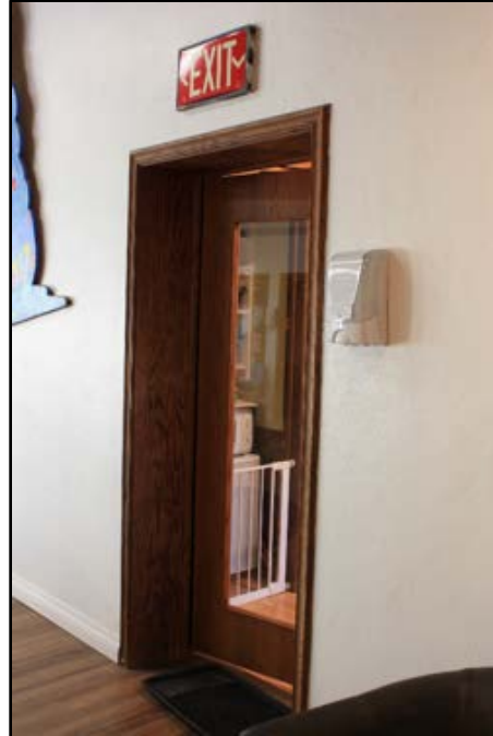
Photo 27 of 54. Entrance to the east addition in the original concrete block wall of the east elevation of the Mexican Branch meetinghouse. Camera facing northeast.
