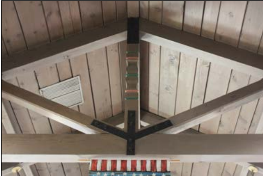
Photo 25 of 54. Detail of truss and wood ceiling in the chapel of the Mexican Branch meetinghouse.
