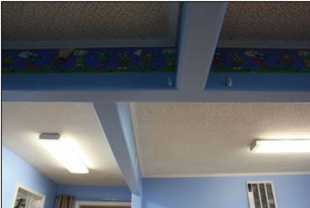
Photo 43 of 54. Detail of the ceiling where walls have been removed to create an open plan space in the Mexican Branch meetinghouse. Camera facing south.
