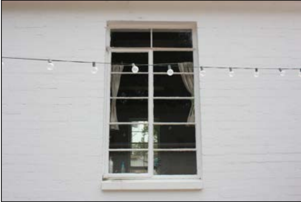
Photo 15 of 54. Detail of original two-by-four casement window with transom in the west elevation of the chapel in the east wing of the Mexican Branch meetinghouse. Camera facing east.
