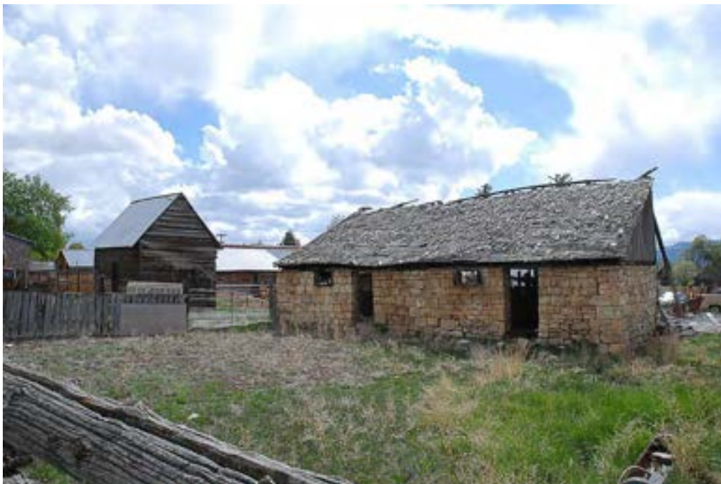
Photograph 38 Stone barn (right) and log granary (left) at 87 E. 200 North. Camera facing southwest.
