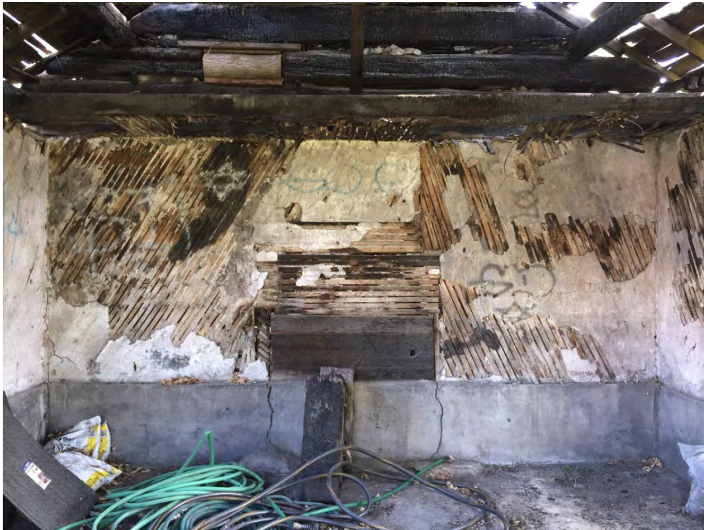
4 of 6. Interior view of south wall of cabin BEFORE. Camera facing south.
