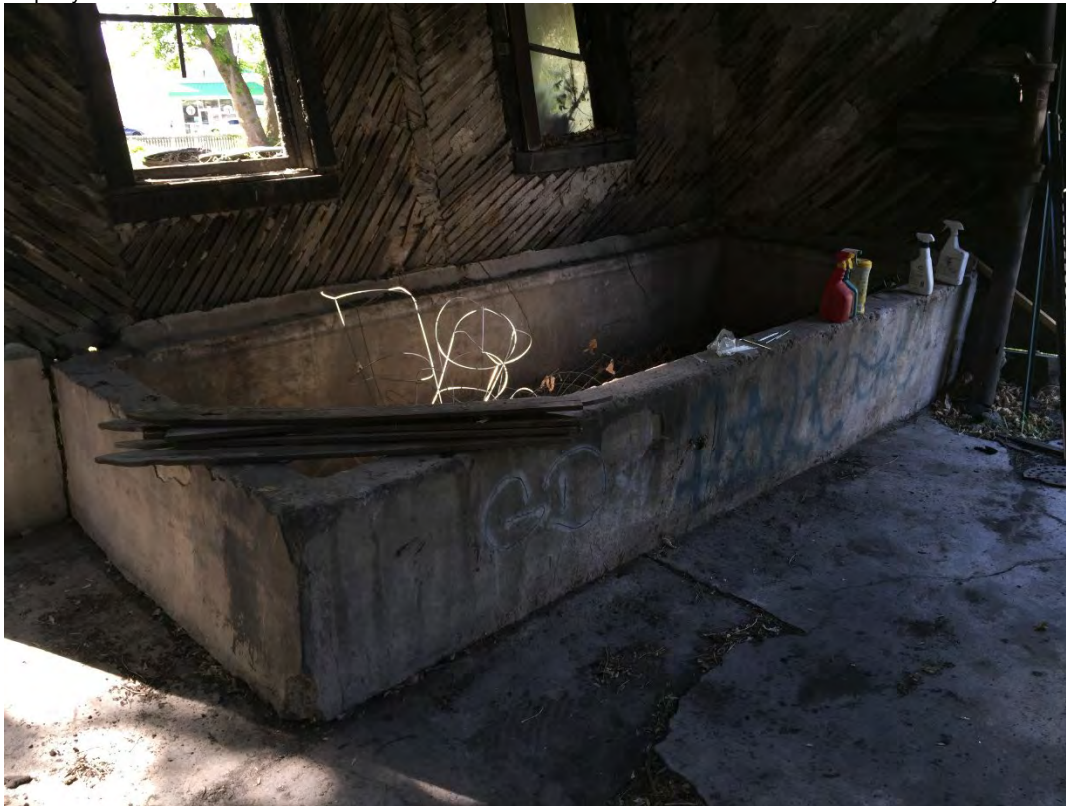
5 of 6. Interior view of NW corner of cabin- BEFORE. Camera facing NW.
