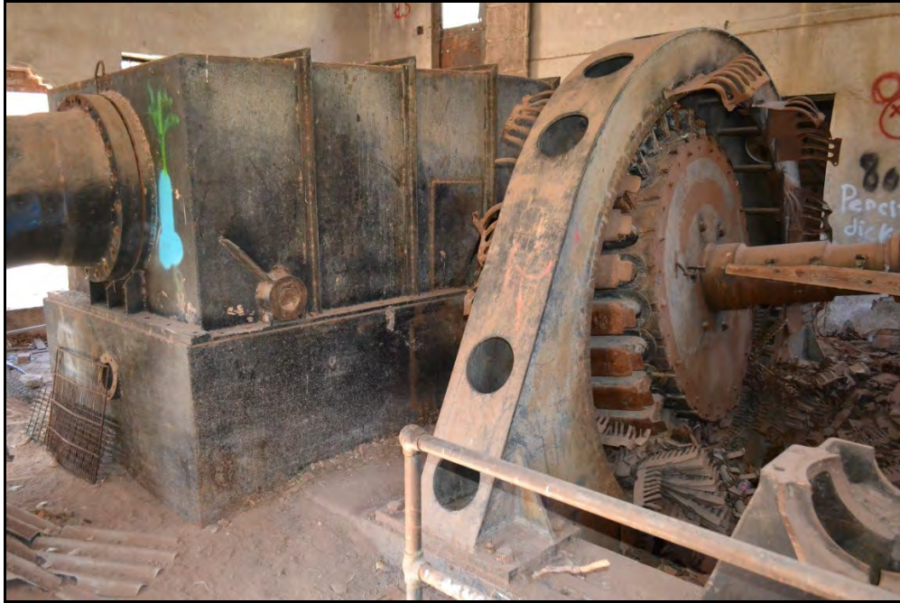
20 of 29. Turbine and Pelton wheel casing. Camera facing northwest.
