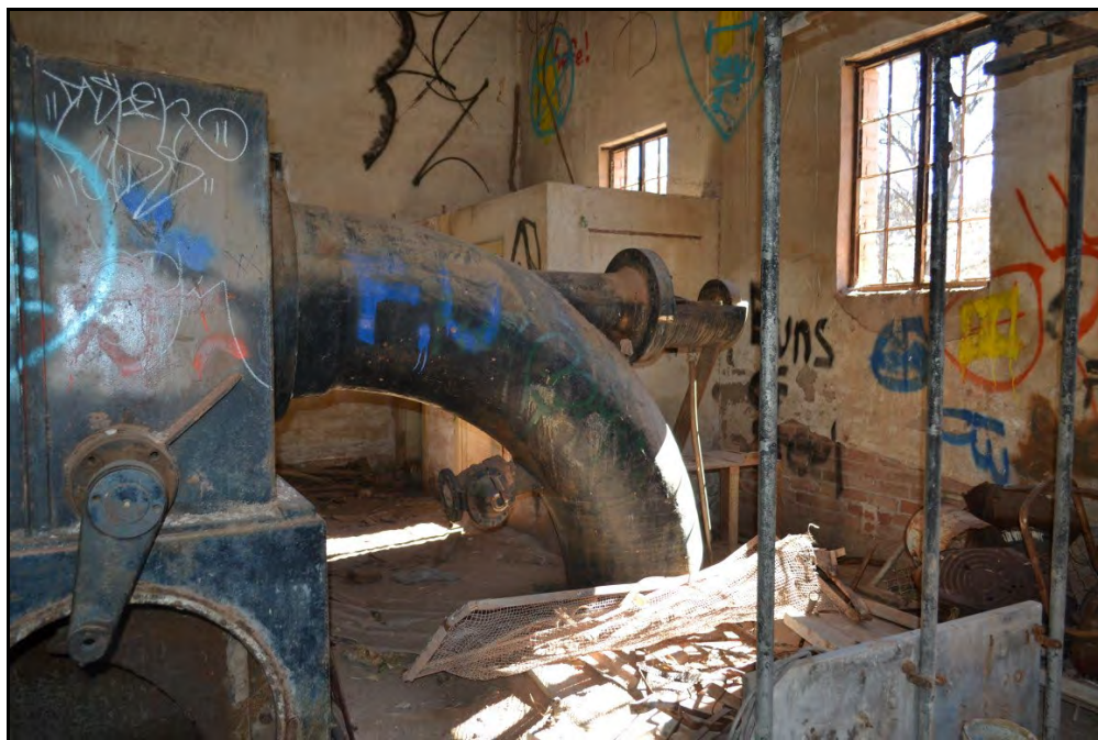
19 of 29. Partial view of Pelton wheel/penstock and south wall. Camera facing southeast.
