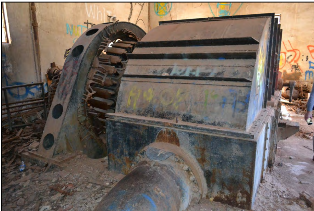
21 of 29. Pelton wheel casing and turbine. Camera facing southeast.
