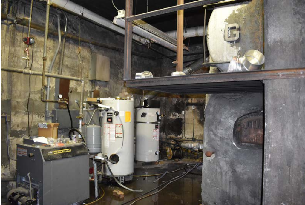
21 of 42:Boiler room in the basement of the hotel. Camera facing southeast.
