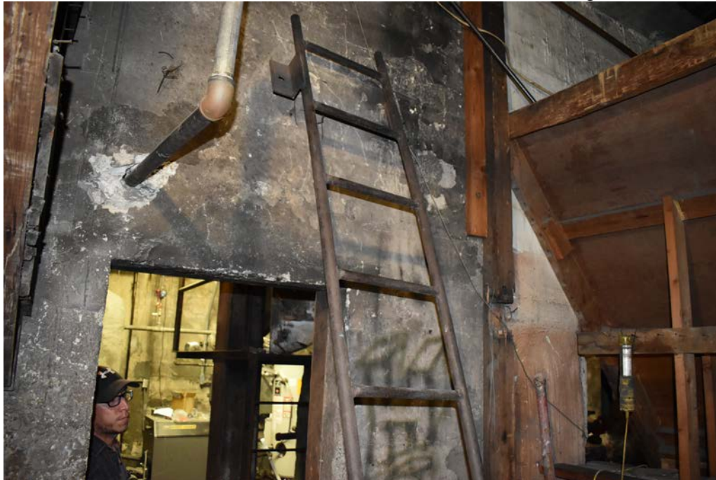
22 of 42: Boiler room in the basement of the hotel. Camera facing east.
