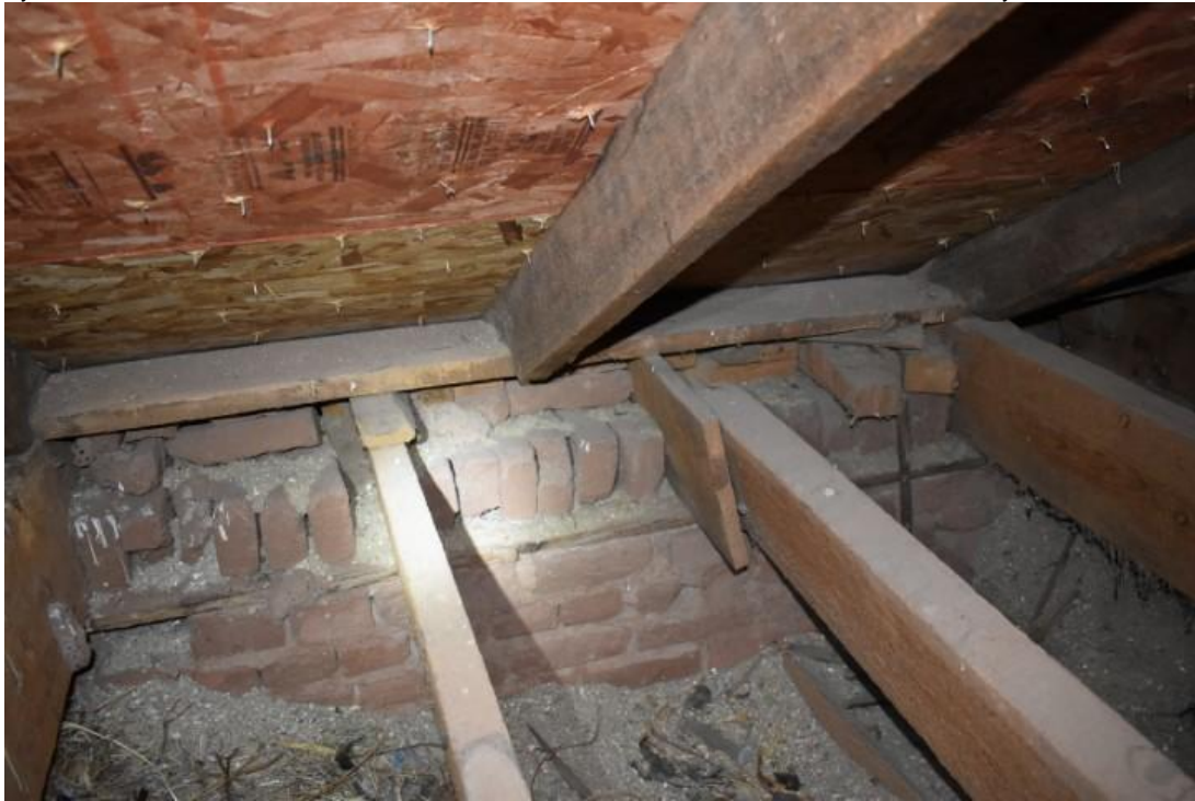
Photograph 13 of 20 Roof truss, plate and brick construction 1867 section. Camera facing north. (Photo Steven Cornell)
