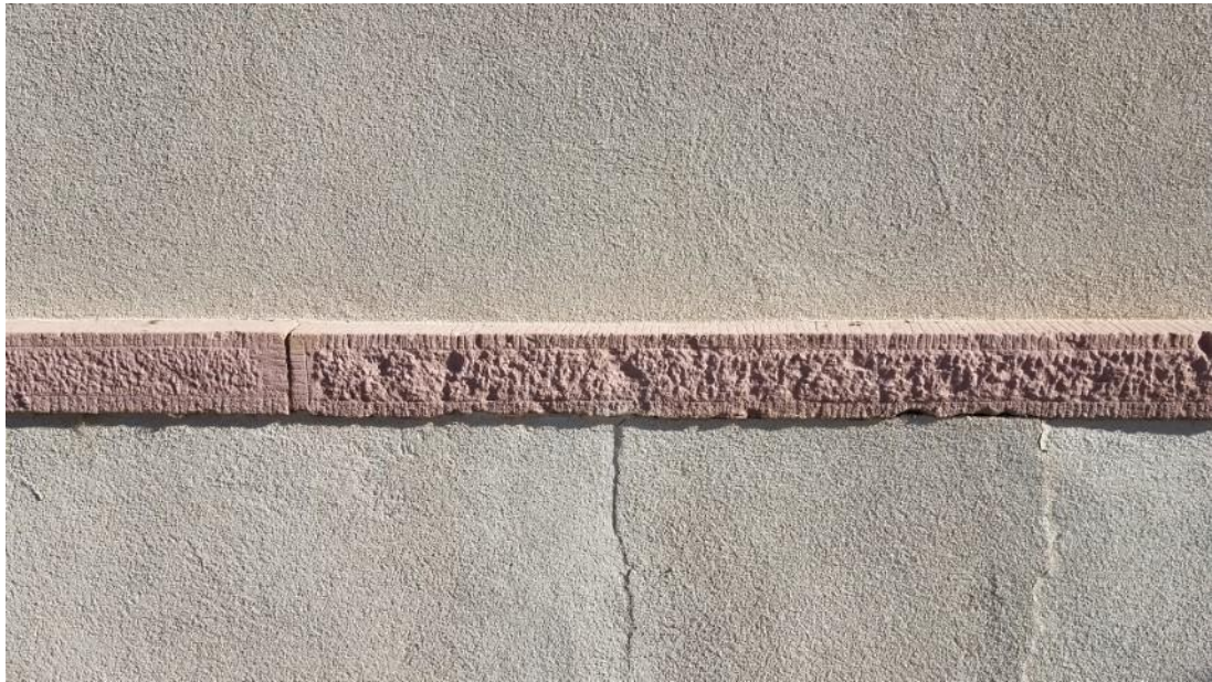
Photograph 9 of 20 Water table stonework detail on 1879 section. Camera facing north. (Photo August 2019)
